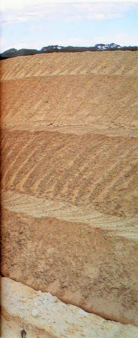
Drain dug through Stoneleigh Park, an area of heritage bushland, to carry ground water for discharge into the southern Coorong.
